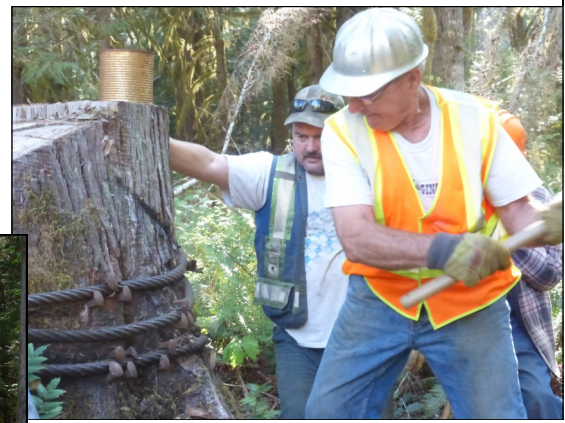
(Below) Eric Netzer spikes the nose guy line to the anchor stump after the nose of the Heel Boom was raised.
