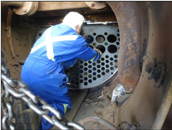
(Below) The front Tube Sheet is hung ready to be welded while Brent was finishing welding the Tube Sheet at the other end of the Boiler.
