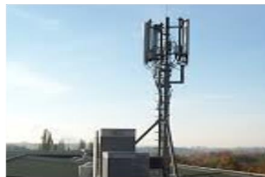
Non-Penetrating Mount — Rooftop
