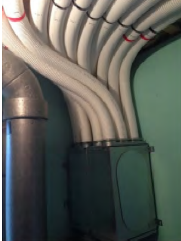
Fig. 4.4 Mixing box (above HRV not shown), with home run ducting (HDPE with smooth interior surface). Image courtesy of NZ Builders.
