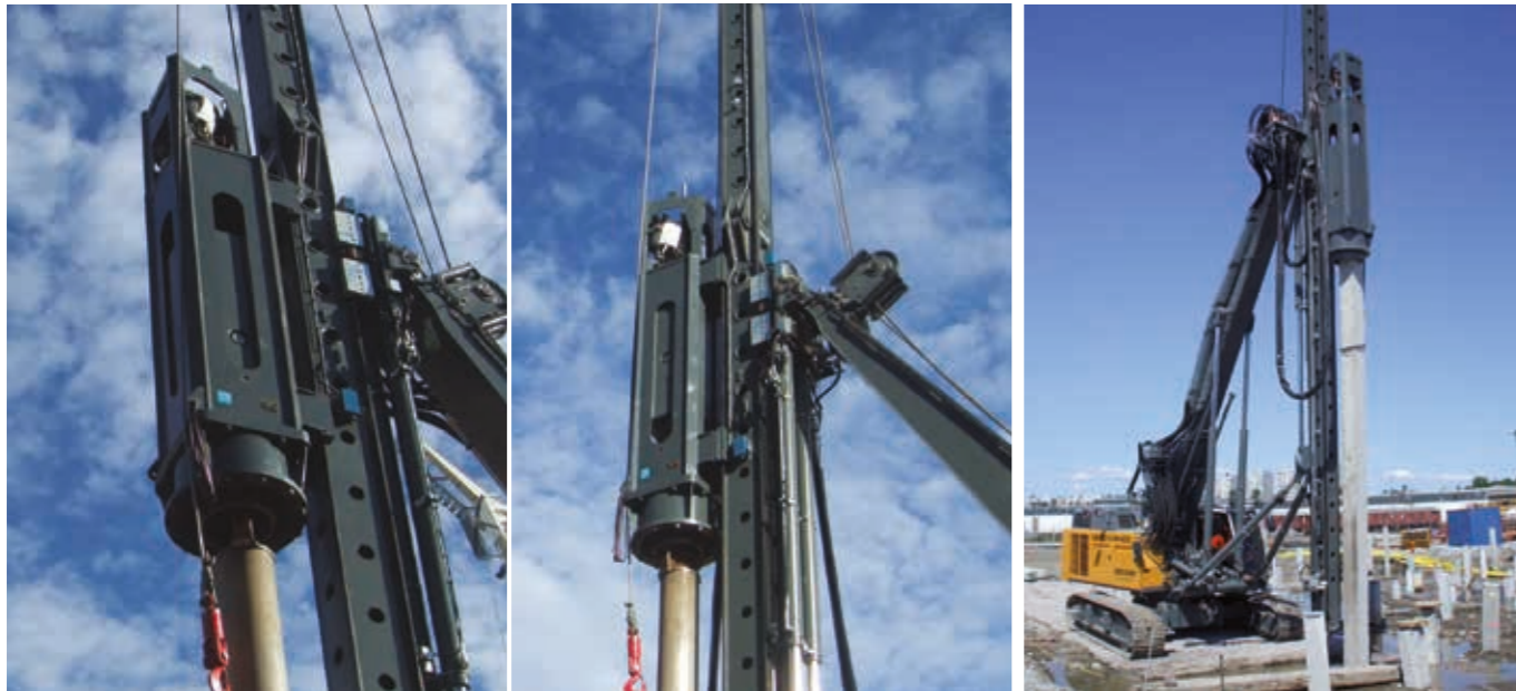
ABOVE: THE LIGHTWEIGHT LX HAMMER GIVES GREATER STABILITY TO PILING RIGS, ESPECIALLY IN APPLICATIONS WHERE A GREATER REACH IS REQUIRED.
