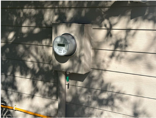
Electric Service Into House
