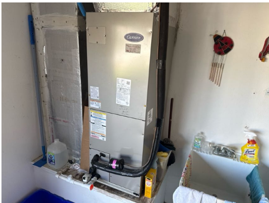
Furnace/ Air Handler 1
