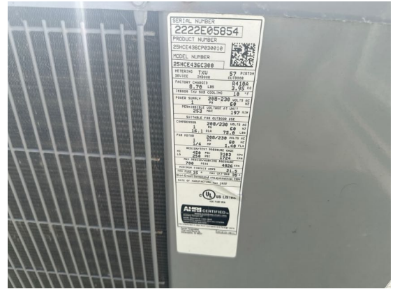
Maufacturer's Label - Compressor 1
