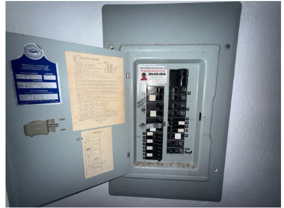
Main Electrical Panel
